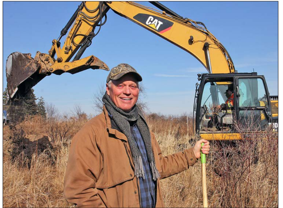
Ducks Unlimited Canada volunteer Phil Holst (foreground) was instrumental in the creation of the Tribe family wetland, here under construction courtesy of Nick Sweazey, right, in the high hoe.
